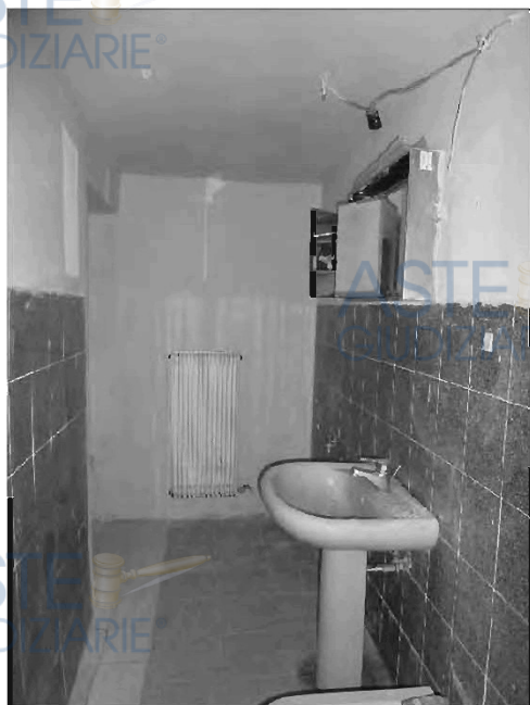
Locale bagno piano terra
