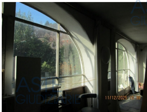
Camera condonata al piano seminterrato
